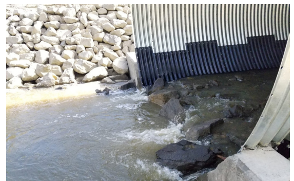
Outlet End View
